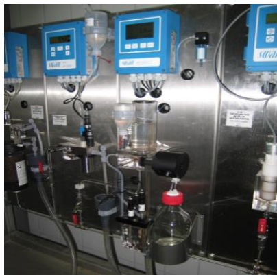
Fig. 4. Appearance of mounting rack PE92 with installed chemical analysis devices
